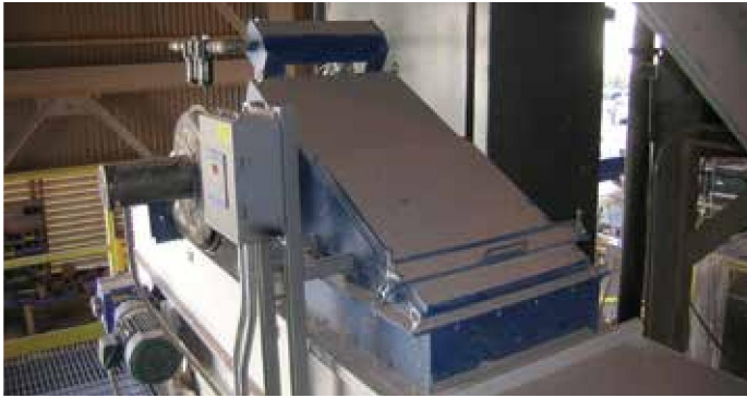
CPV-2 - Weigh belt feeder with limestone dust 800 cfm (1,359 m 3 /h)
